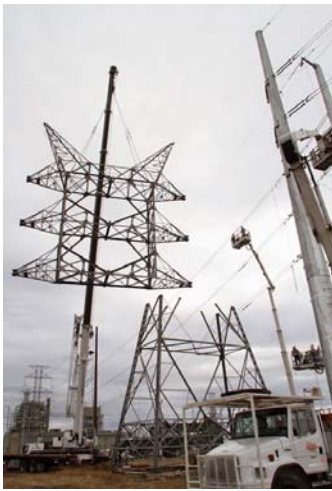
Transmission Circuit upgrades
