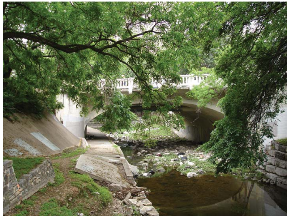
The path beneath the Red River Street bridge near Palm Park has eroded into the creek.
