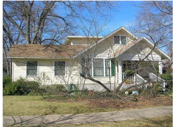
This incompatible side addition is flush with the front of the original house.
