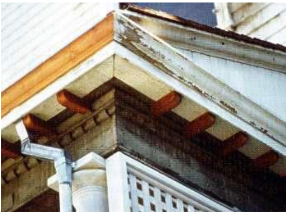
Damaged exterior wall materials can be repaired or replaced in-kind, as in the fascia board to the left.
