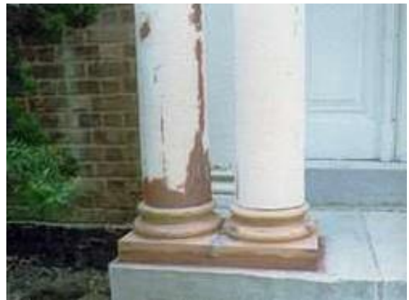
Deteriorated wood porch elements can be repaired in place with epoxy consolidants and fillers.
