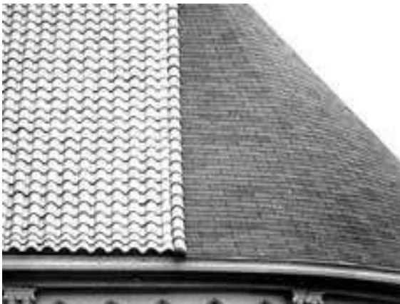
Asphalt shingles are an incompatible replacement substitute for the original Spanish clay tiles.
