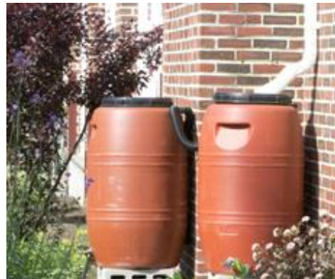
Rain Barrels connected to gutters
